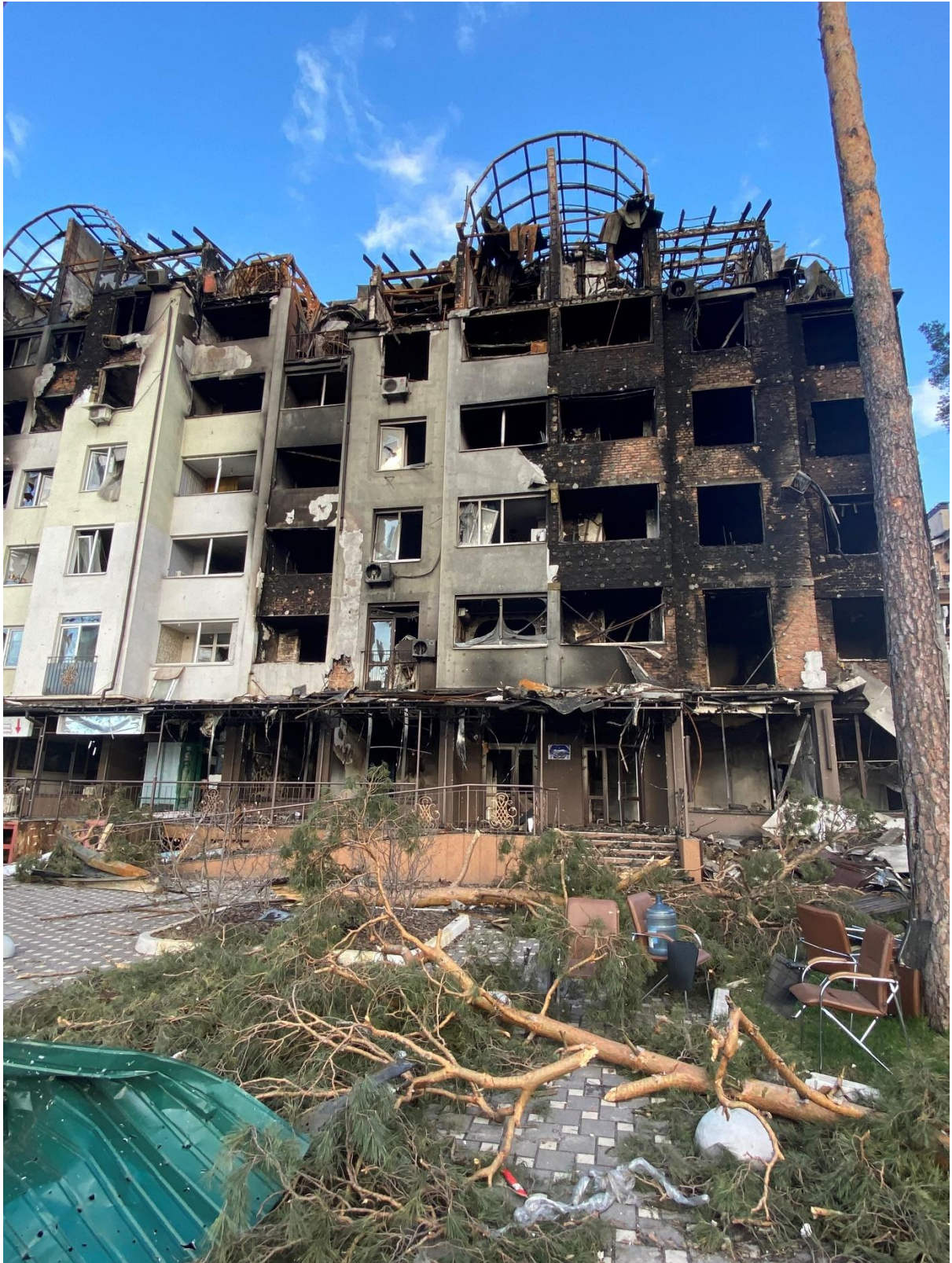
Destroyed residential buildings in Irpin
